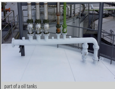
part of a oil tanks
